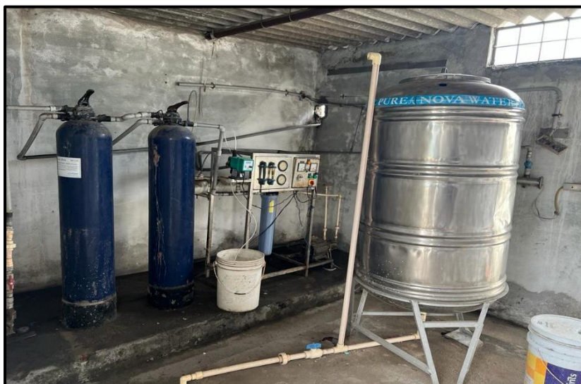
Water management activities – R.O Units in Sri Indu College of Engineering & Technology
