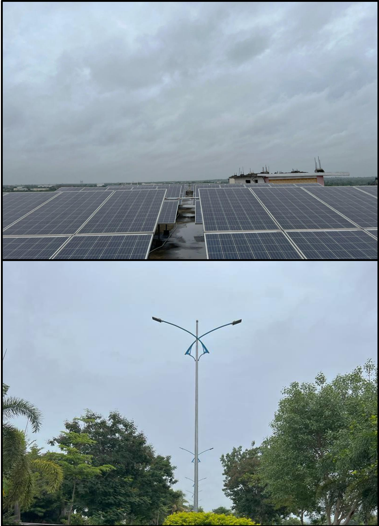
Solar Panels Observed at the SICET Campus, Telangana
