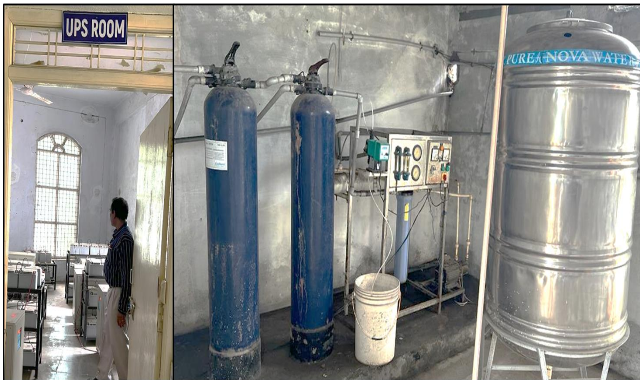
UPS Room and RO Water Facility available in the Sri Indu College of Engineering & Technology, Telangana
