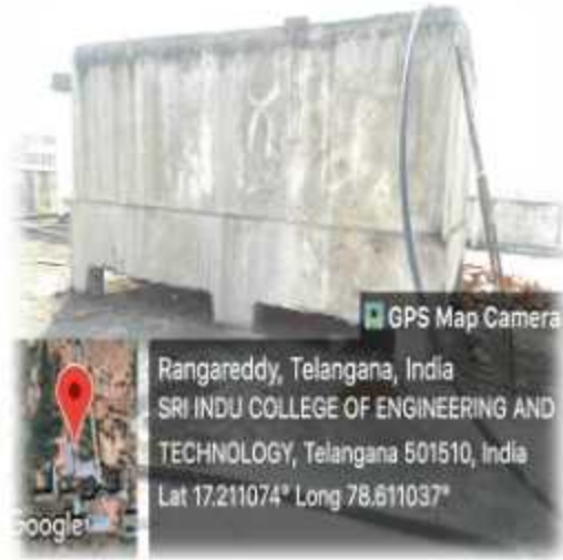
Storage of water in tanks
